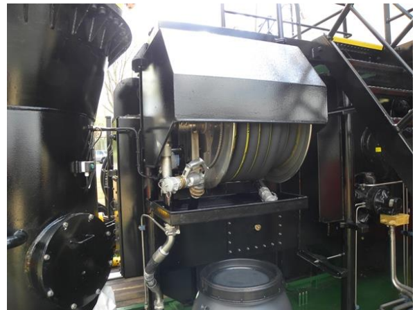
Fuel supply winch
