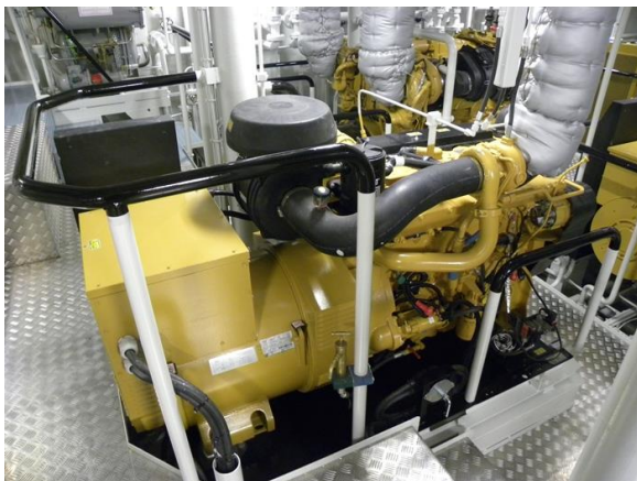
One of the two Caterpillar generator sets
