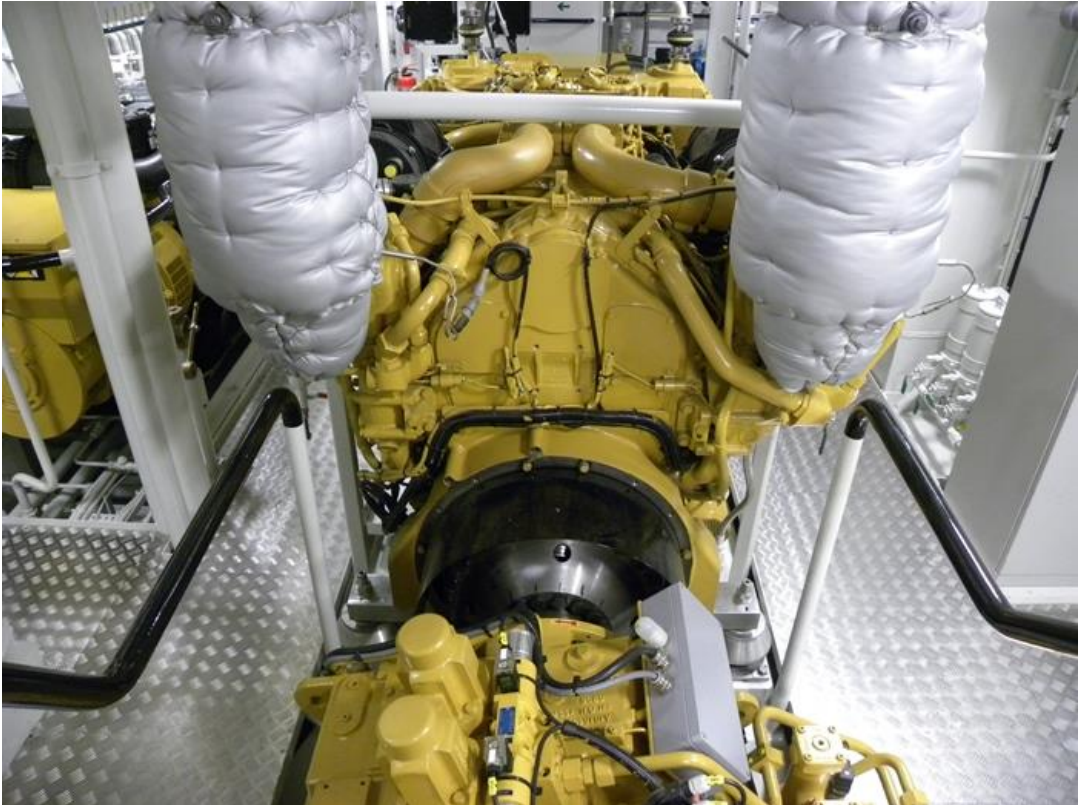
Centre Caterpillar Engine gearbox view
