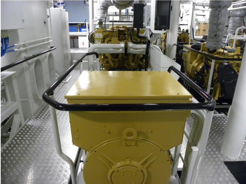
Centre Caterpillar E-generator view
