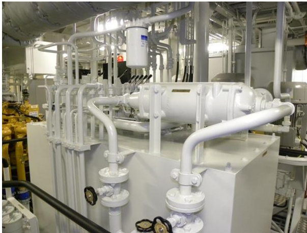
Hydraulic powerpack unit
