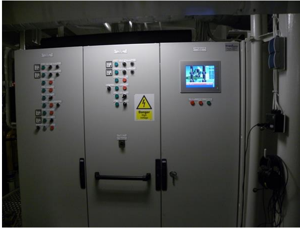
Electric power distribution board
