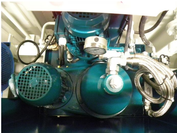
Fuel oil separator
