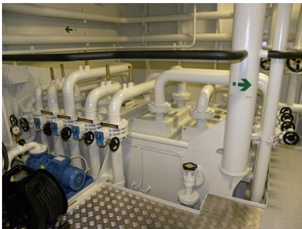
SB side main engine coolingwater coolers
