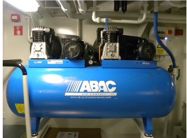
Air compressor set
