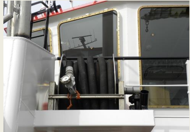
Fuel supply winch
