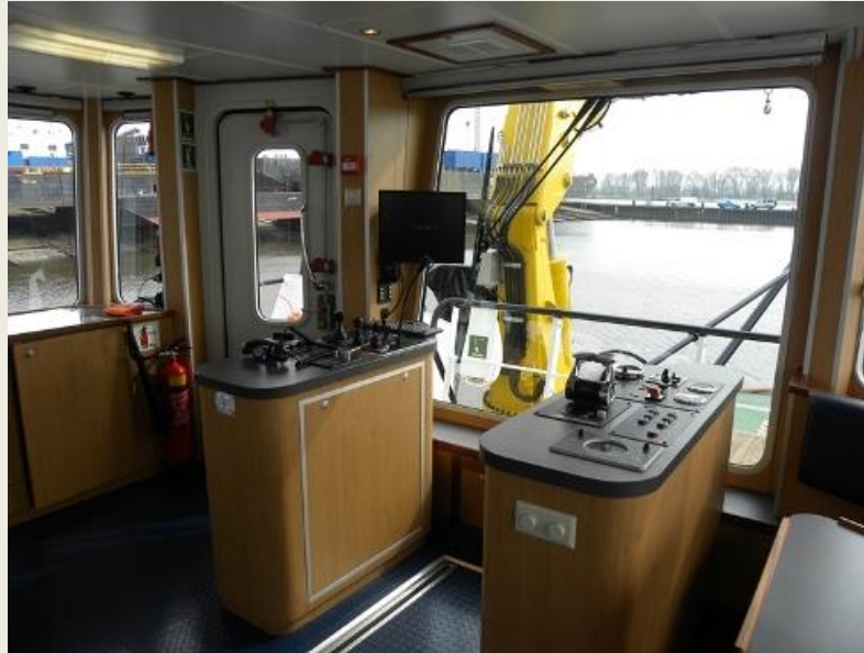
Aft bridge manoeuvring winch control console
