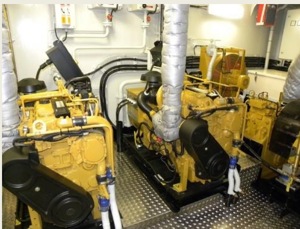
Two Generator sets
